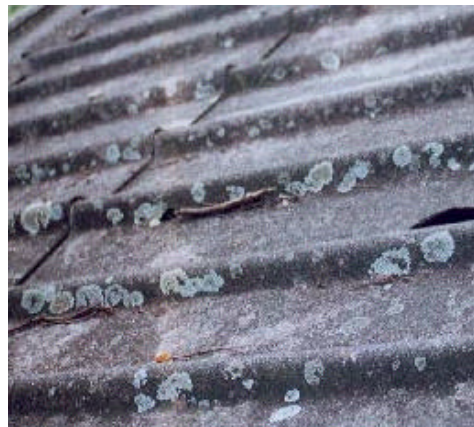
Lichens growing on asbestos
